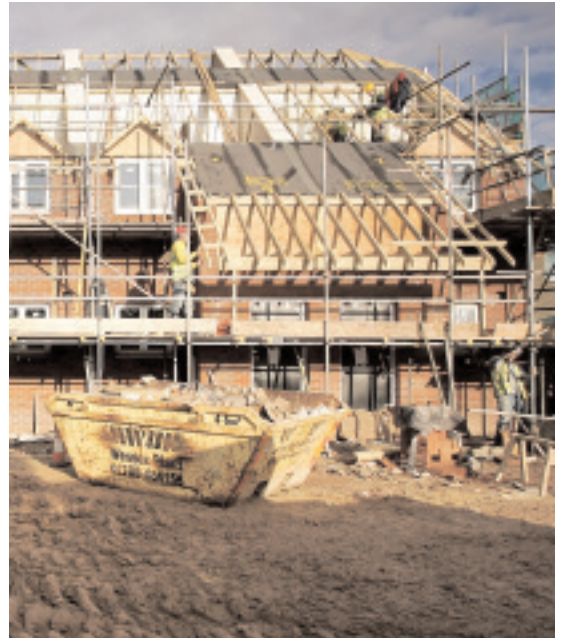
Using a single skip for all waste types is a missed opportunity to implement good practice
