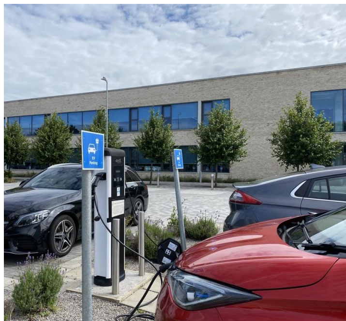
Image 9: Electric vehicle charging facilities at Forth Valley College, Falkirk Campus (image credit: Lara Fahey, EAUC, 2023).
